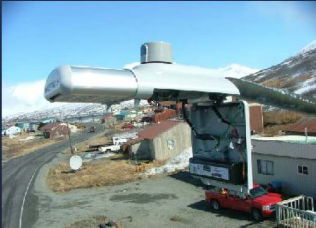
King Cove: LED Light Fixtures
