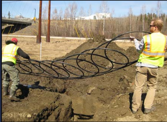
Fairbanks Ground Source Heat
