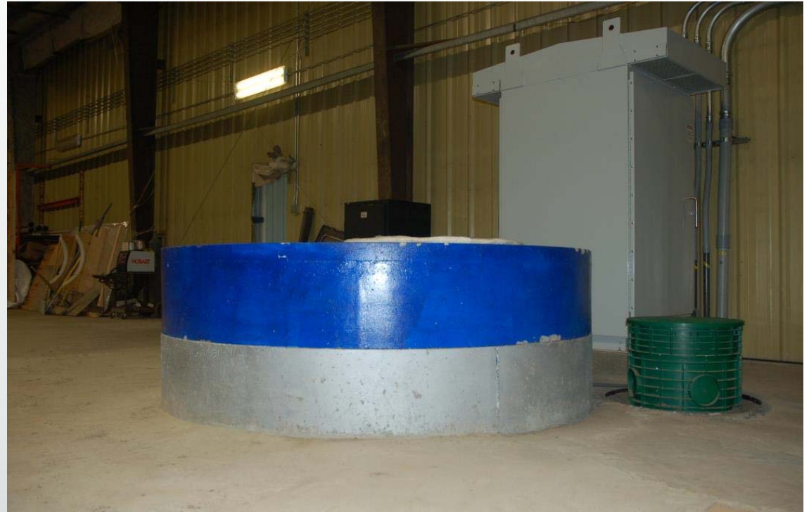
TDX St. Paul Flywheel Project
