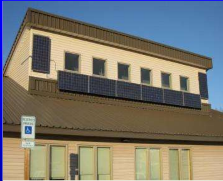
Solar PV system
