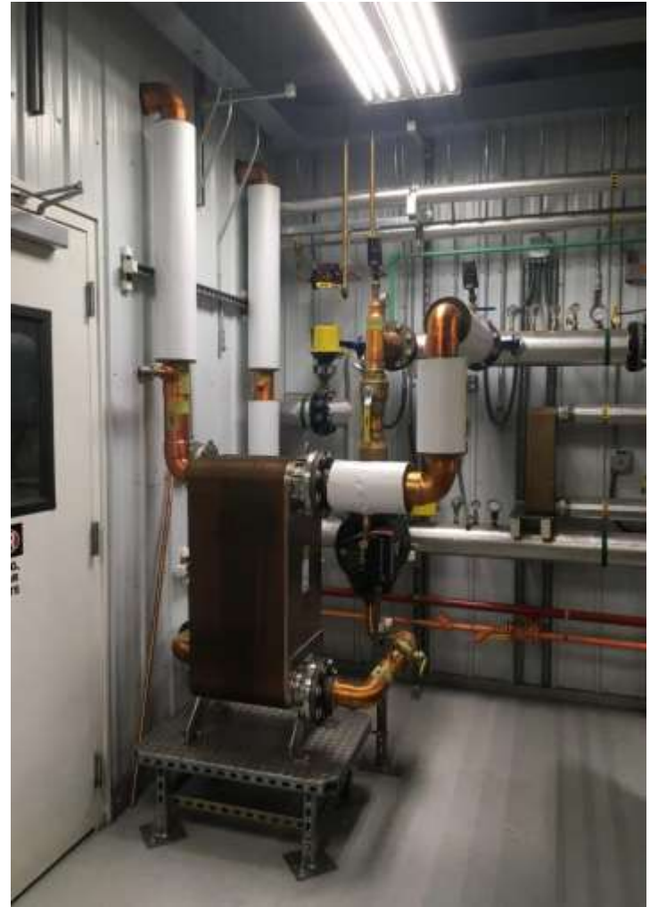
Flat plate heat exchanger in AVEC's Stebbins Power Plant.
