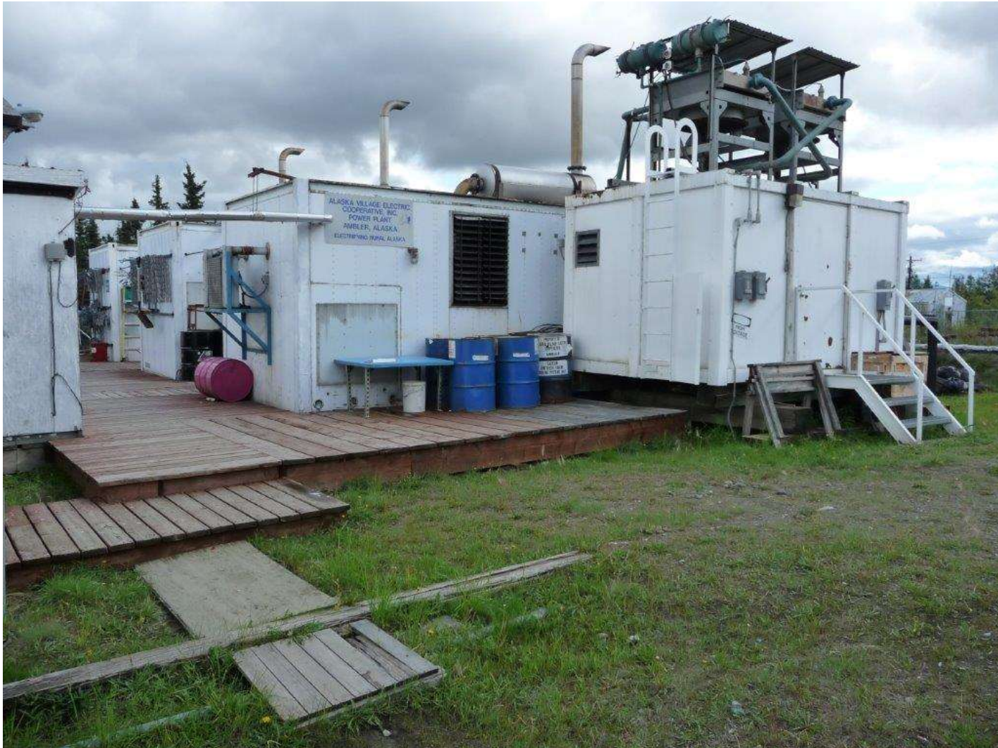
Ambler Power Plant with HR Module
